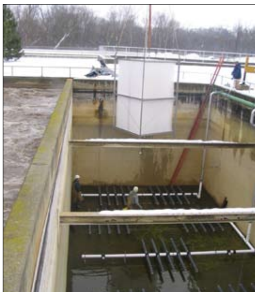
The Village of Mukwonago (Wis.) Wastewater Treatment Facility turned to fixed-film activated sludge treatment instead of building additional aeration tanks for nitrogen removal.
